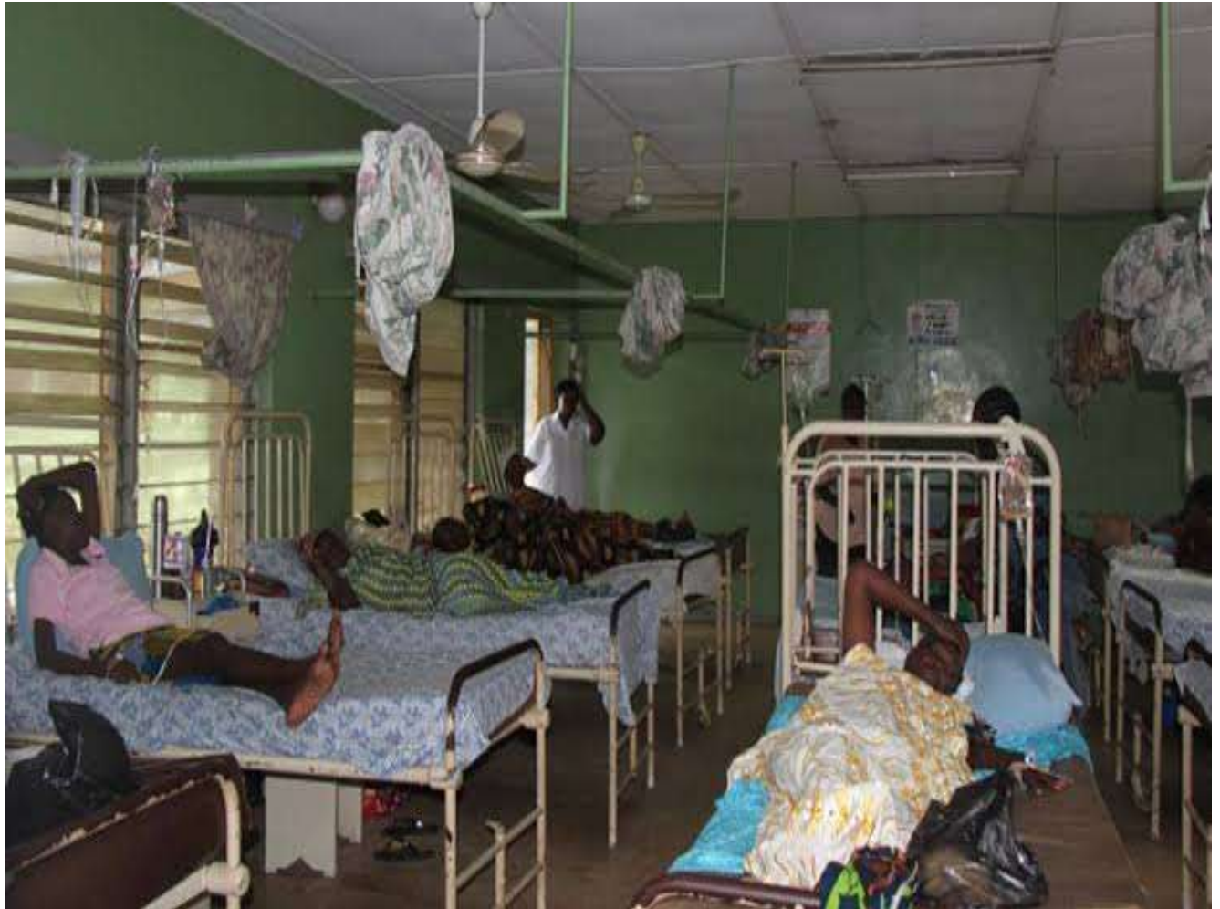
Plate 2: Showing poor circulation of spaces at the wards; this leads to congestion and discomfort to both patients and staff.
