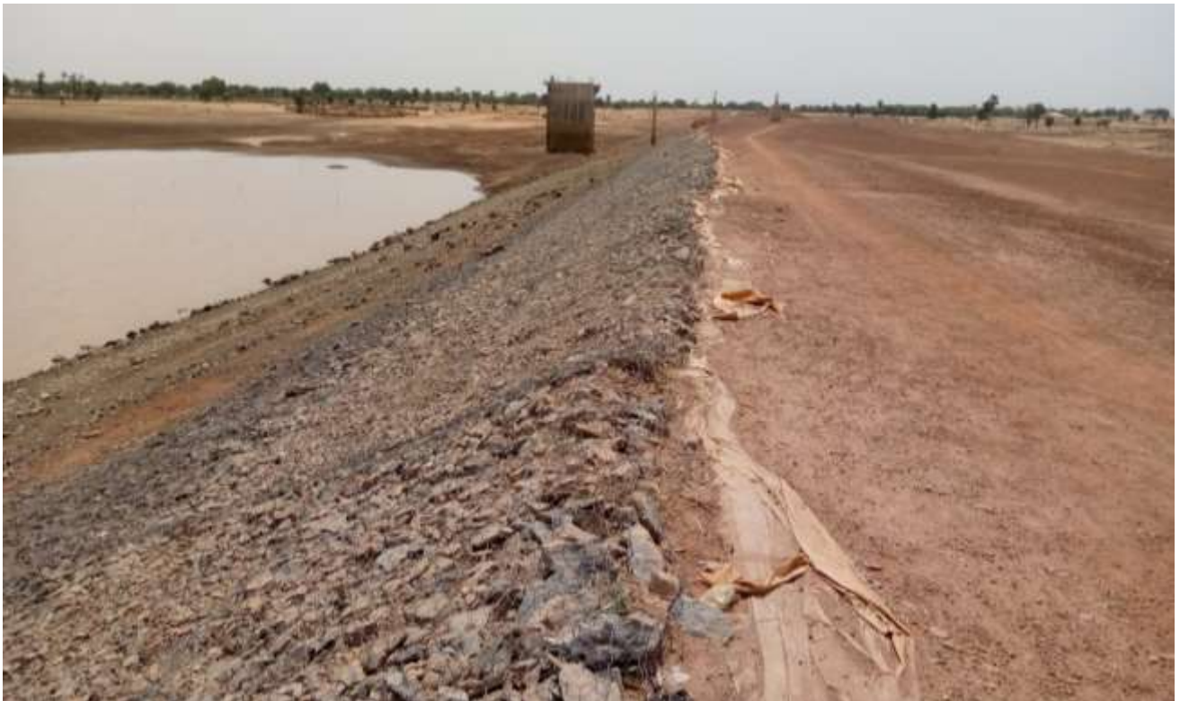
Figure 2 : Dallaje dam site showing the uncompleted nature of the dam.
