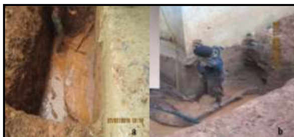
Fig 2: Foundation probe showing (a) the column base at the left hand side of the building (b) the measurement of foundation depth
