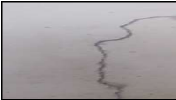
Fig. 5: Vertical crack observed on first floor internal wall of the project structure.
