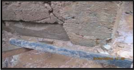
Fig. 6: punching shear failure on foundation column
