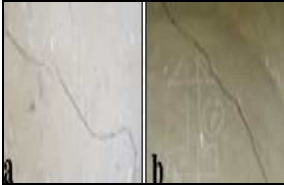
Fig. 4: Some of the observed cracks, (a) diagonal crack on ground floor internal wall (b) diagonal crack on ground floor external wall
