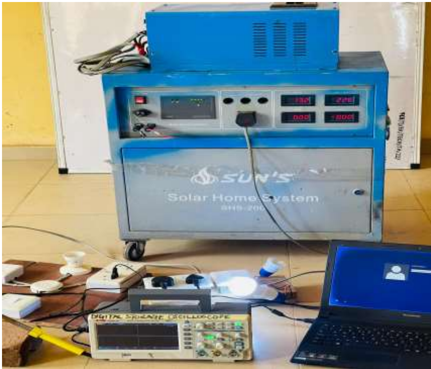
Figure 3: Final output stage demonstrating stable power supply from the integrated DC Battery and Solar Inverter System .
