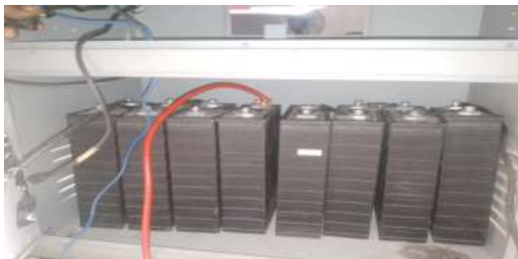
Figure 1: LiFePO 4 batteries Connected in series and parallel
