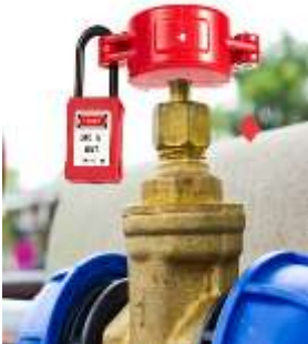
Fig 2.4 Lock-Open and Lock-Closed Systems Valve (slb.com, 2022)
